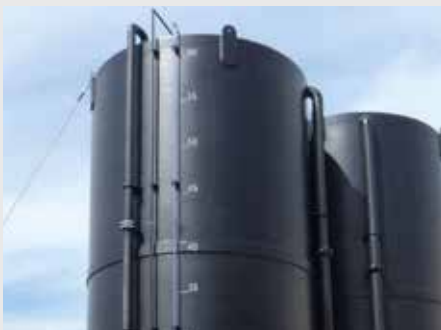
Storage tanks made of polyethylene
